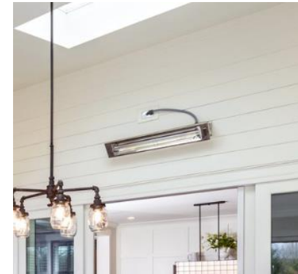
Outdoor Heaters Pre-Wires
